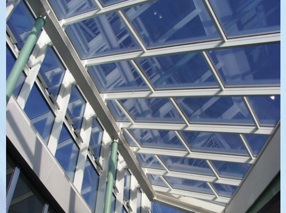
Charter School, Dulwich Automatic Shaped Head Smoke Vents
