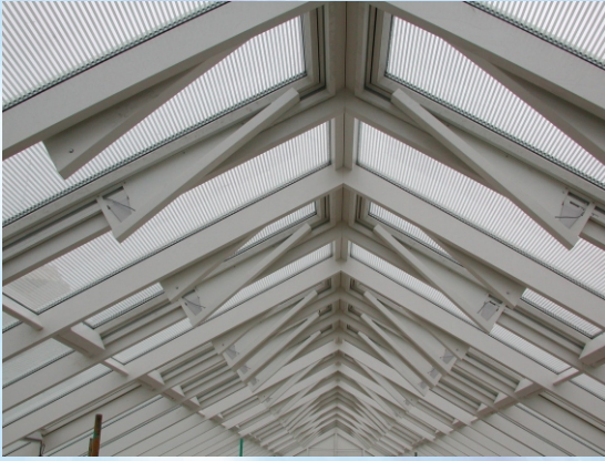
Fulham Broadway, London SSP1 Automatic Roof Smoke Vents
